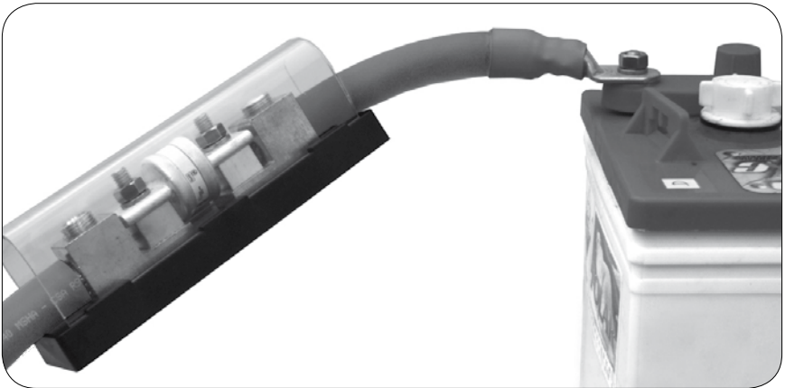
Fig. 3.20. Positive cable connection to the battery – with Class "T" Fuse Assembly
