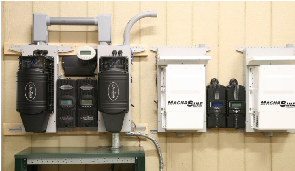
OutBack and Magnum horizontal stacked systems
