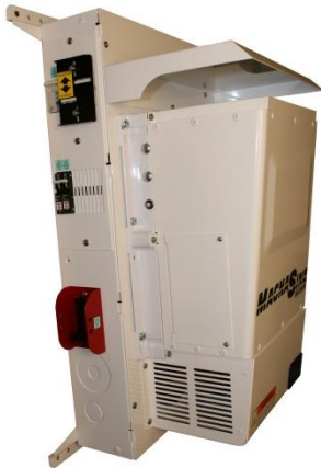
Left Hand Magnum as installed
